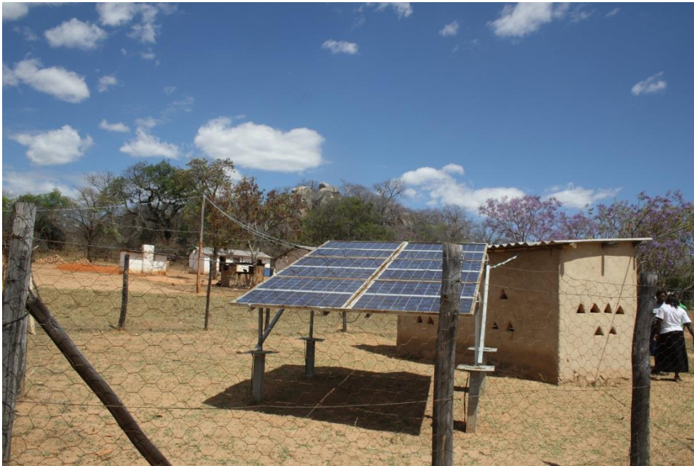
Figure 8: Solar Powered Mini-grid at Chitora Secondary School, Mutare.
